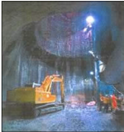
Turrella ventilation shaft
