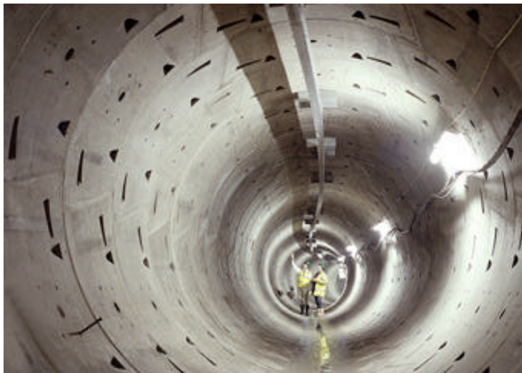
Figure 4: Inside the completed tunnel from Cricklewood to Canons Corner. National Grid's 20 km Elstree to St John's Wood cable tunnel was constructed within a 12-month period using three (3) tunnel boring machines.
