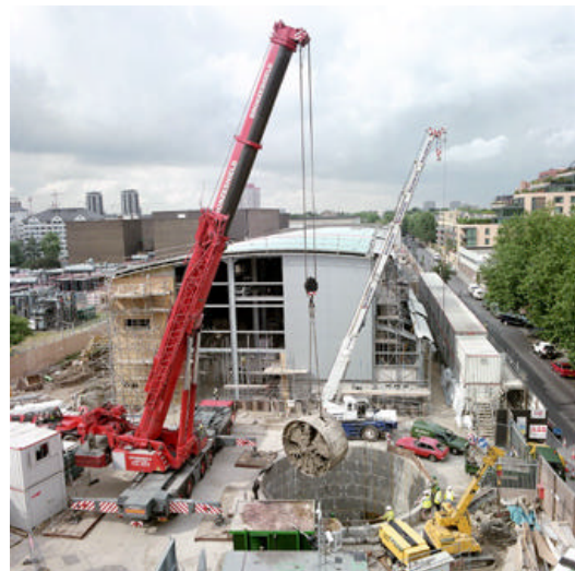
Figure 5: Construction of the new 400 kV substation and removal of the Tunnel Boring Machine after completion of the section of tunnel from Cricklewood to St John's Wood.
